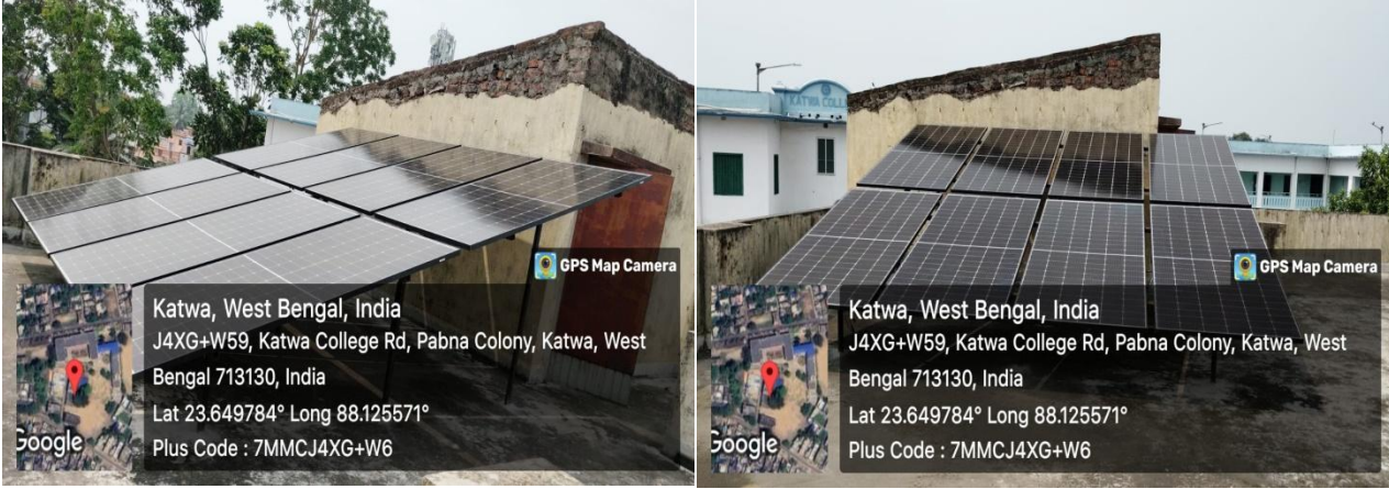
Rooftop Solar Panel on the Administrative Building of Katwa College
