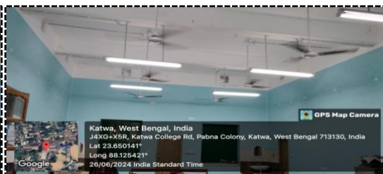
LED facility in the staff room
